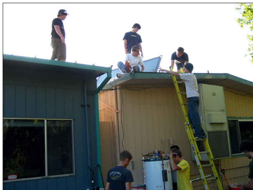
Figure 3. Freshman service learning project with a California K–6 charter school to install a solar water heater. Cal Poly students conducted a user needs assessment and identified the engineering design constraints and requirements to provide hot water to school children to wash their hands and for the science teacher to conduct experiments. They then installed the system and still maintain it. Photo by K. Chen.
