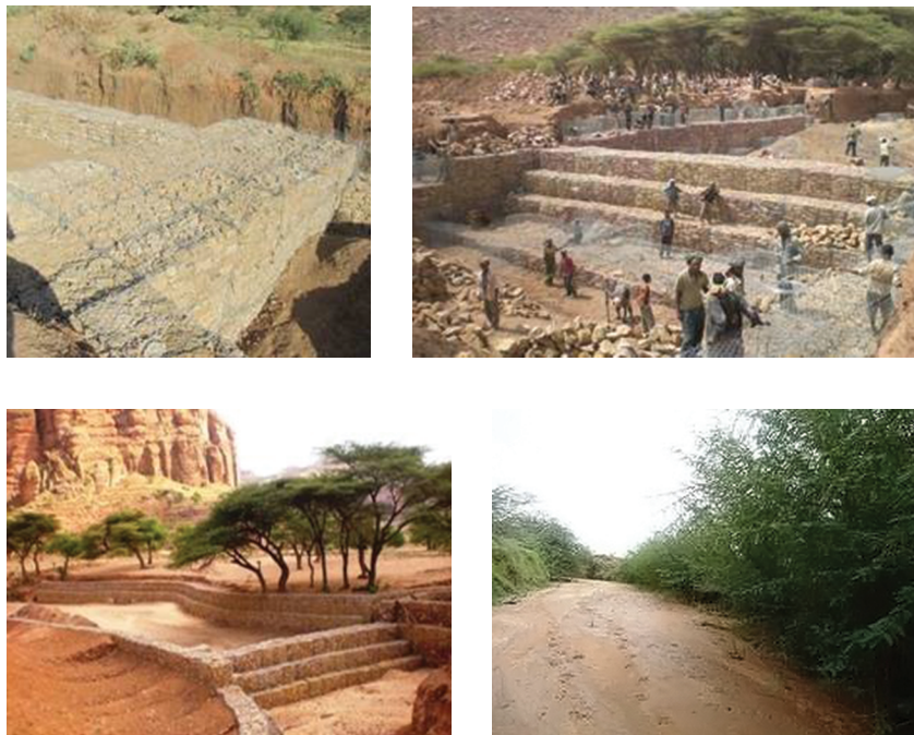
Fig. 6.25 A stone check dam constructed with gabions in Koraro. Top left: gabions. Top right: construction. Bottom left: the finished dam, which is narrower because the gabions penetrate sideways into the gully wall. Runoff flows over the center of the dam. Bottom right: sediment is deposited behind the dam, which can be planted with useful trees like Sesbania sesban along the sides.
