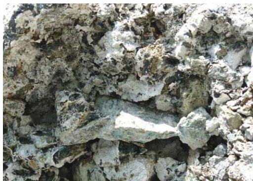
Figure 1: Example of hydromagnesite incrustation at Montecastelli
