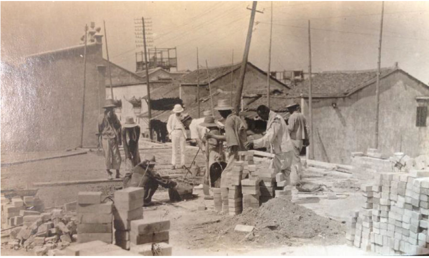
Figure 10. Walter A. Taylor on the construction site of St. Andrew's Church, Wuchang, China. Source: RG251, box 3, Special Collections, Yale Divinity School Library.
