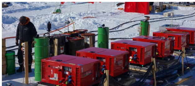
Fig. 4. Main generator bank of the drill system. Note the raised fuel supply drums providing positive pressure to the generator fuel pumps.
