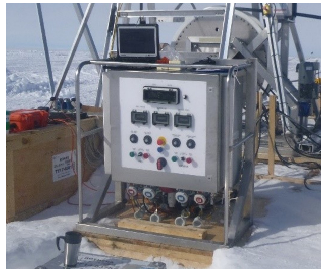
Fig. 9. Winch control panel positioned in front of winch tower during drilling operations with Toughbook computer displaying drill-monitoring data.
