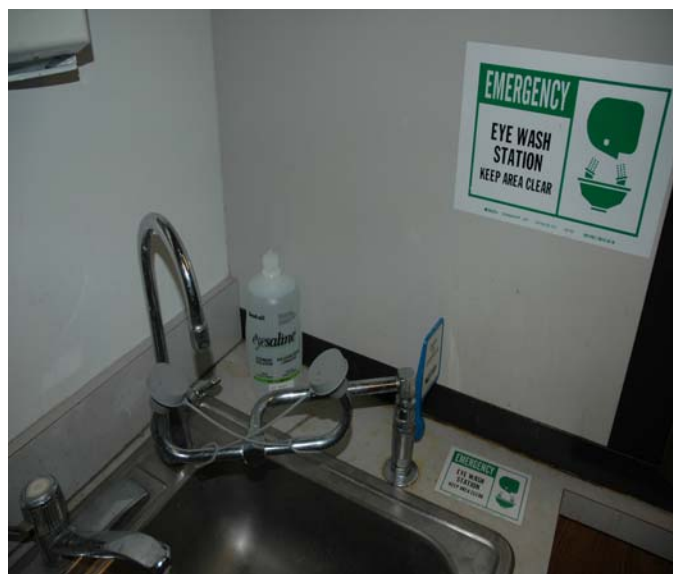
Figure 4 Emergency Eye-Wash Station
